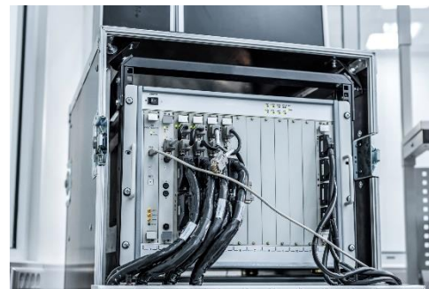
Control panel on test equipment
